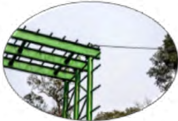
Figure 17.2d. Iron ropes providing approach way to the bridge. Photo credit: Sonali Ghosh
