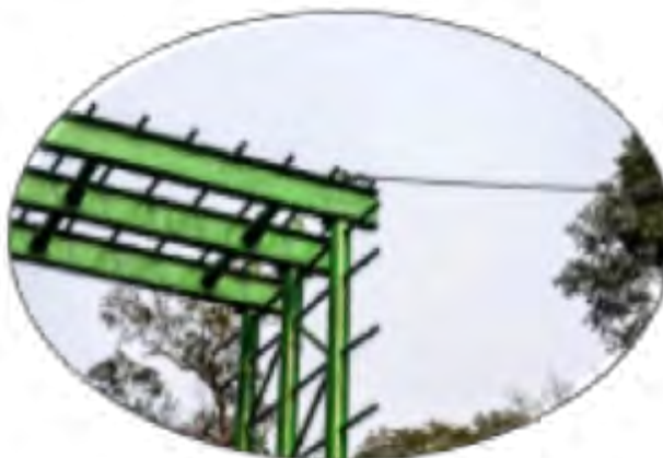
Figure 17.2d. Iron ropes providing approach way to the bridge. Photo credit: Sonali Ghosh
